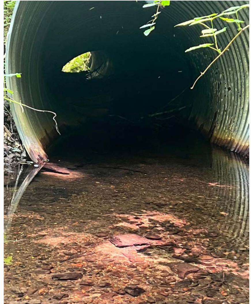
A large culvert in Hubbard Creek shows signs of instability, with both bend and a broken section in the center of the road fill. Failing culverts like this present a significant risk to source water quality.
