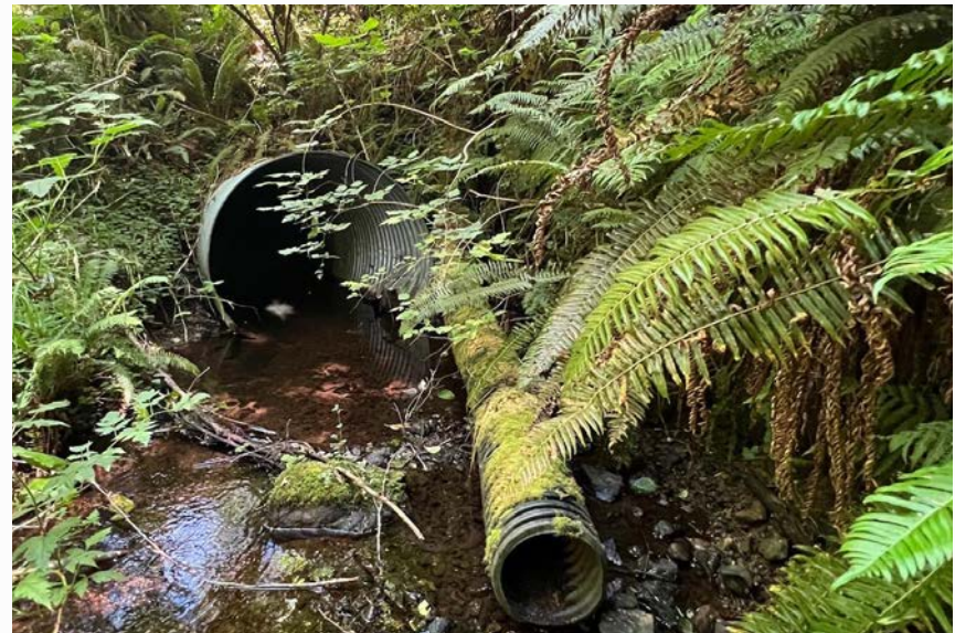
Culvert on the access road from Vista Drive showing odd drainage structures and partially failed primary culvert in Hubbard Creek.
