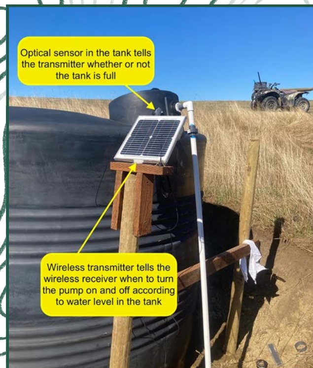
Photos showing an offstream water system using wireless technology to control the pumping of water to a storage tank. In this system, the storage tank is nearly 1,800 feet away from and over 200 feet in elevation higher than the pump.
