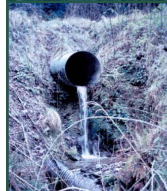
Figure 1: A perched culvert found during a road survey in Lobster Creek in 1997
